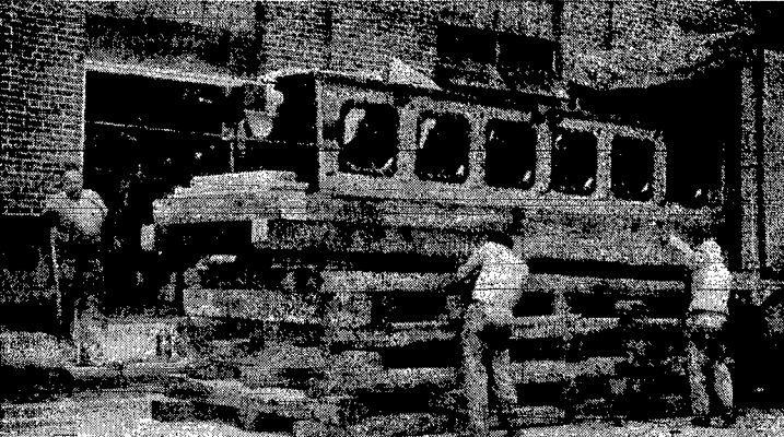
WORKMEN WEDNESDAY were busy dismantling the 14-ton base from the trailer which transporting the Worthington generator engine at the light plant, preparatory to installing the new engine base shown above. In this picture, taken last Wednesday, workmen are shown inching the 14-ton base from the trailer which transported it from Buffalo, N.Y. Company representatives here said improvements developed since the engine was installed would be added before it is put back into operation.
